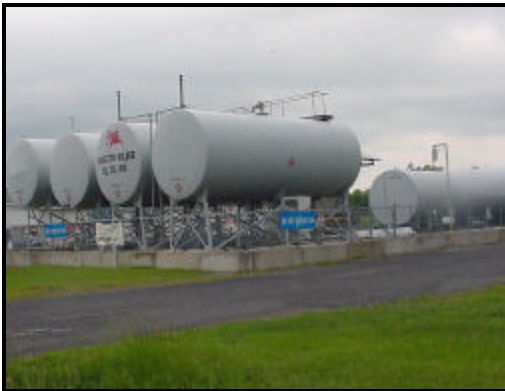
Above ground gasoline storage tanks in Moravia.
