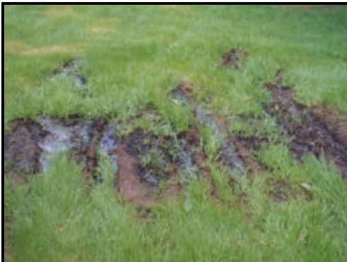
Failing septic tank.
