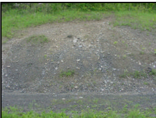
Roadbank erosion along Rockefeller Road.
