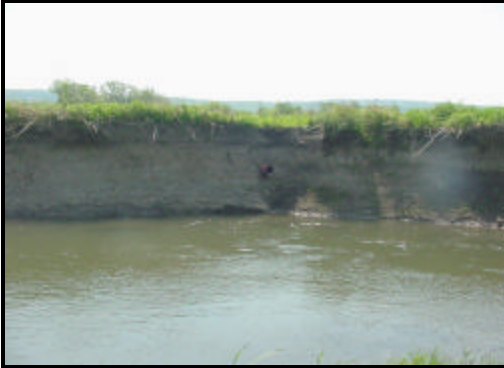
Streambank erosion on the Owasco Inlet.
